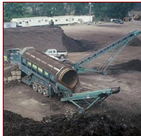
Materials being run through the screener at the NCC White Township facility.
